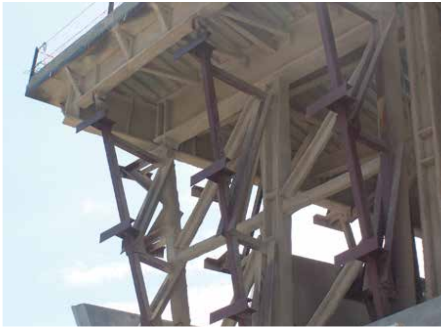
The panels were connected to the structure's steel frame using a connection grid, designated "tree columns," featuring long steel-tube "trunks" with frames branching off. Panels were erected horizontally to allow for horizontal slot windows in selected locations. Many locations didn't allow for traditional vertical panels to be hung and extend floor to floor. Photos: Datum Engineers
