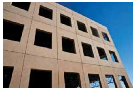
The above photo displays erected, precast concrete sandwich panels insulated with Thermomass System NC.
