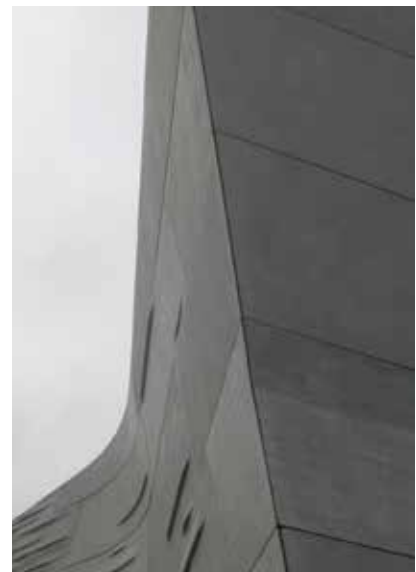
The plinth panels were curved, with most of them canted, radiused, half canted or half radiused. Photos: Gate Precast Co.
