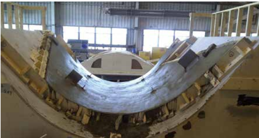
The precaster had to cast a variety of curved panels with many different radiuses, many of them tight. These curves required the back of the panels to be formed up so the concrete stayed inside the form at the panel was cast.
