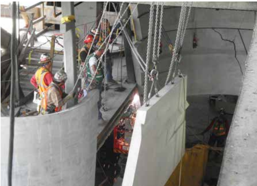
Erection of the panels required meticulous care, often requiring chain falls and cone-alongs to set them. Photos: Gate Precast Co.
