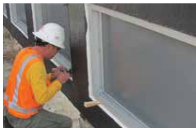
Prior to delivery, each precast panel was pre-glazed, caulked, inspected, and applied with waterproof coating on the back face.
