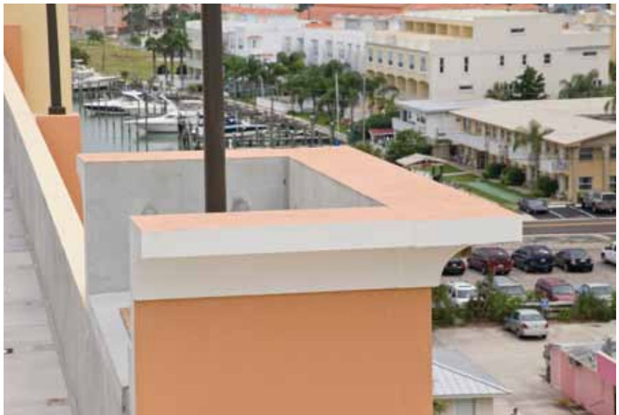
Improved durability and increased erection speed was achieved by integrally casting the cornice into the wall panels.
