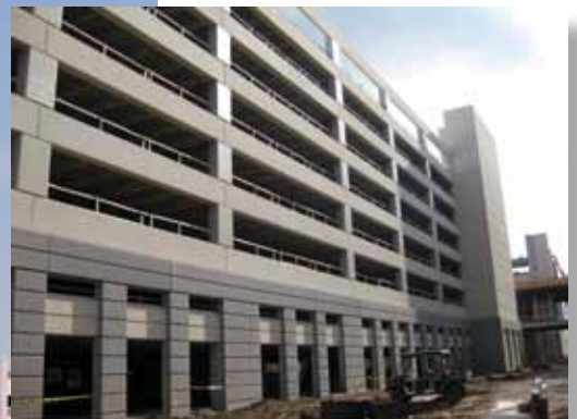
Erection was completed in December on two eight-level, 1,300-car parking structures at the new Veterans Administration Medical Center in Orlando. The exterior finish includes a light sandblast on upper levels with an acid etching to achieve a different texture on column covers.
