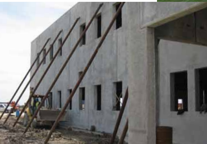
The panels at the Armed Forces Reserve Center were erected in a vertical fashion, facilitating the design of bays and other penetrations.
