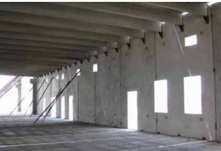
Clear spans were provided for the facilities at the Armed Forces Reserve Center by using 24-inch-deep double tees to span the spaces. The double tees rest on corbels cast into the interior face of the load-bearing precast concrete wall panels.
