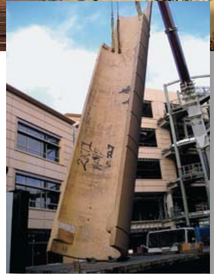
Precast concrete column covers provide a complementary look for the grand trellis, which is supported by 70-ft-high tubular steel purlins.
