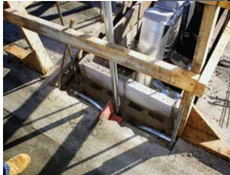
The hollow-core slabs could be erected quickly, thanks to the precaster's ability to continue erection through cold winter weather.
