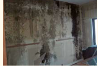
Fig. 1 Appearance of mold on drywall.
