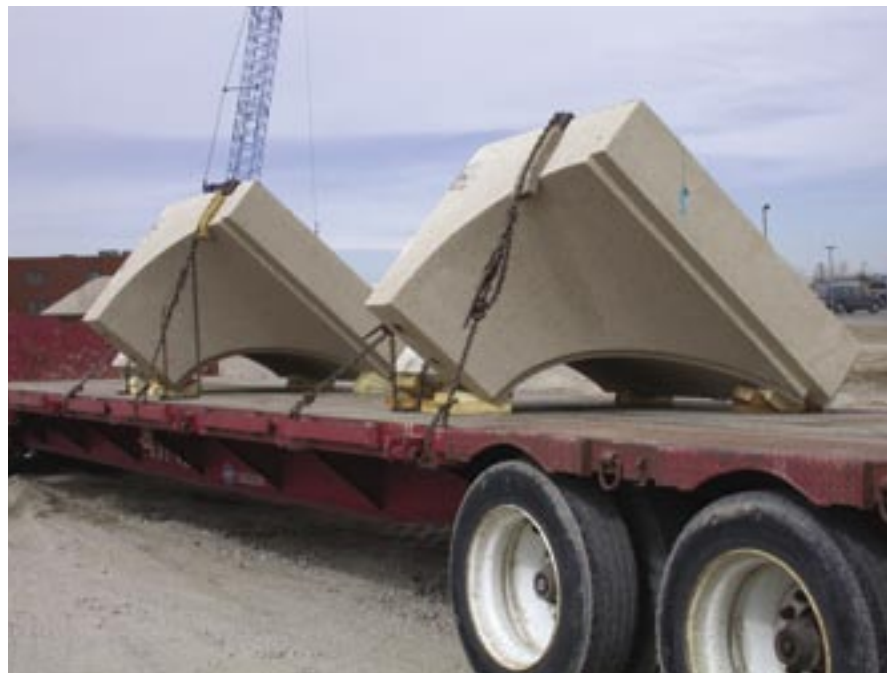
Fig. 16. Trailer bed transport of two curved precast concrete parapet pieces. Production of these projecting parapets required high skill and tight tolerances.
