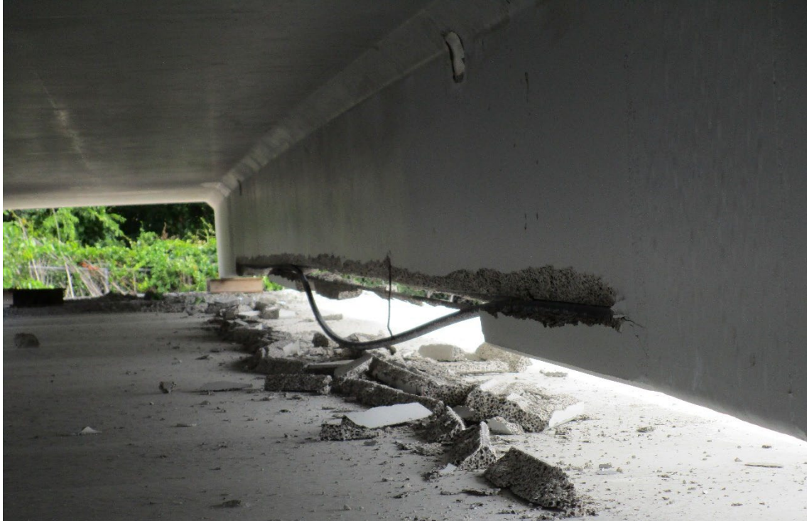
Figure 1 – Failure of double-tee stem due to creep-rupture
