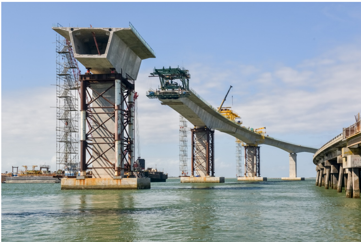
Fig. 8 Navigation Spans construction, showing balanced cantilever construction of the precast concrete post-tensioned segmental concrete box girder superstructure.
