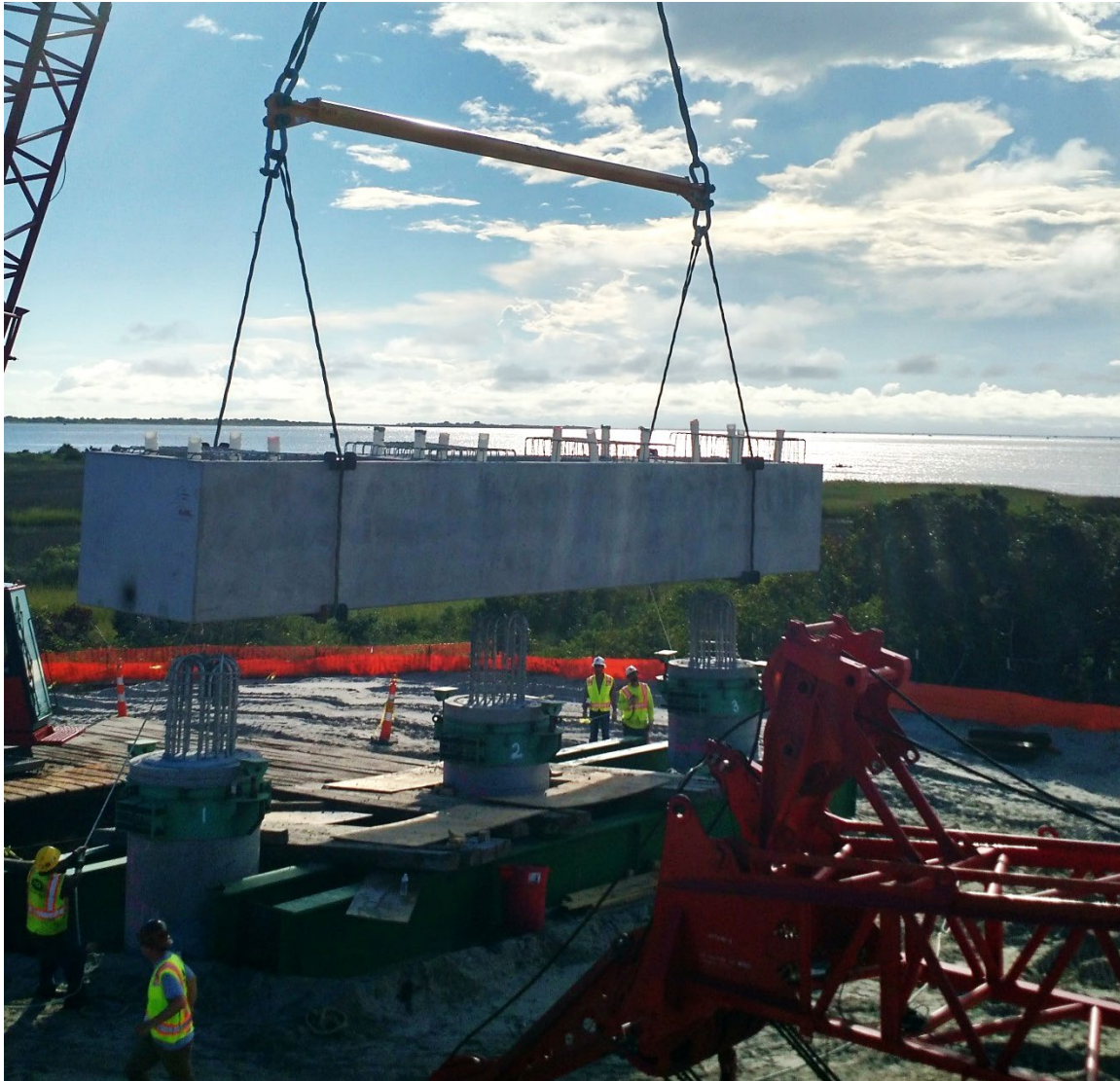
Fig. 3 Setting of the first precast concrete bent cap on 54" diameter precast concrete cylinder piles in the North Approach Spans, creating an all-precast substructure unit.
