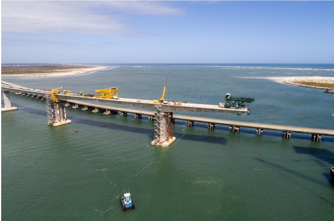
Fig. 9 Navigation Spans construction, showing balanced cantilever construction of the precast concrete post-tensioned segmental concrete box girder superstructure.
