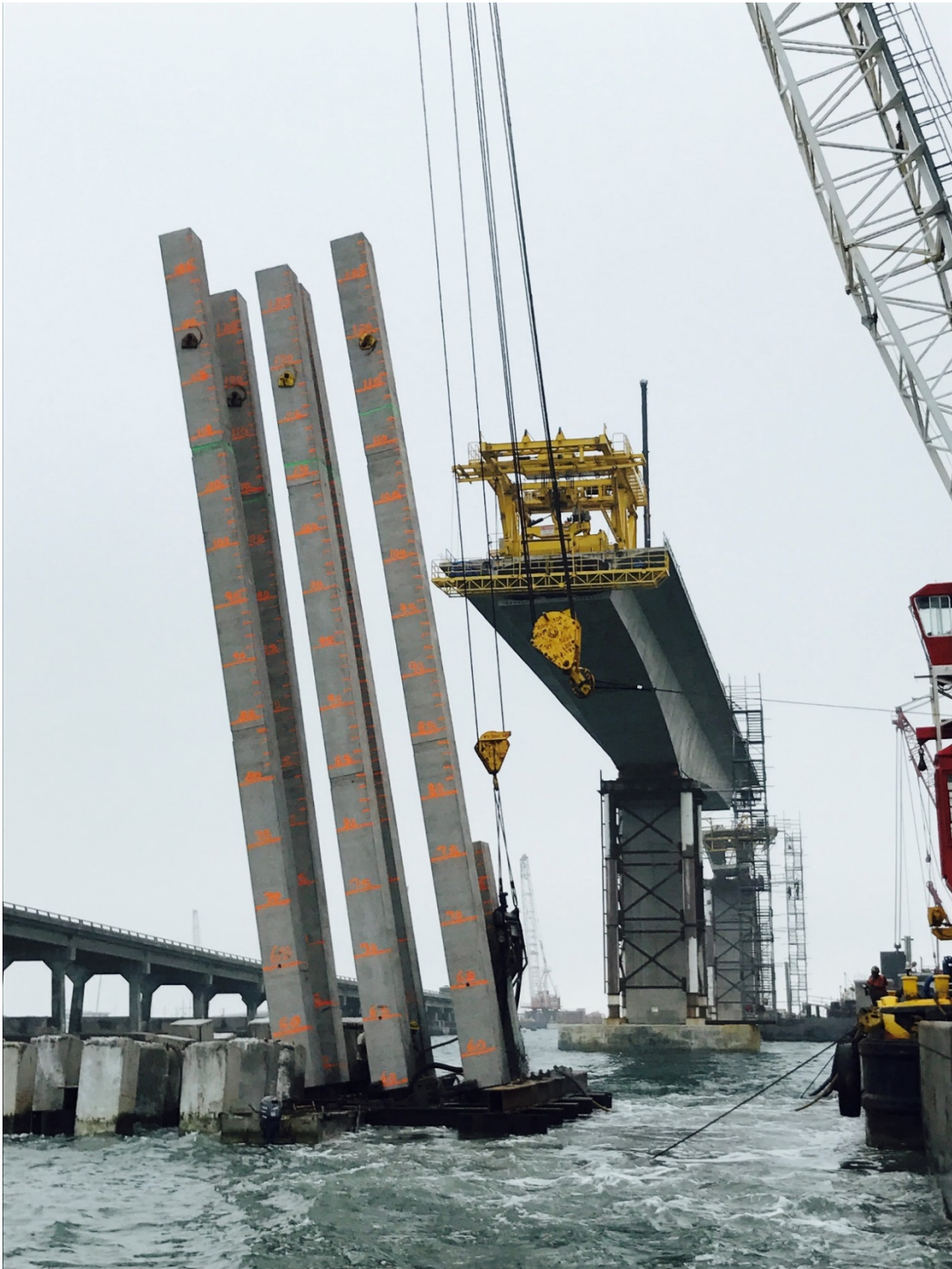
Fig. 6 Navigation Spans construction, showing installation of 36" precast concrete square piles in foreground and balanced cantilever construction of precast concrete segmental box girder superstructures on precast concrete box columns in the background.
