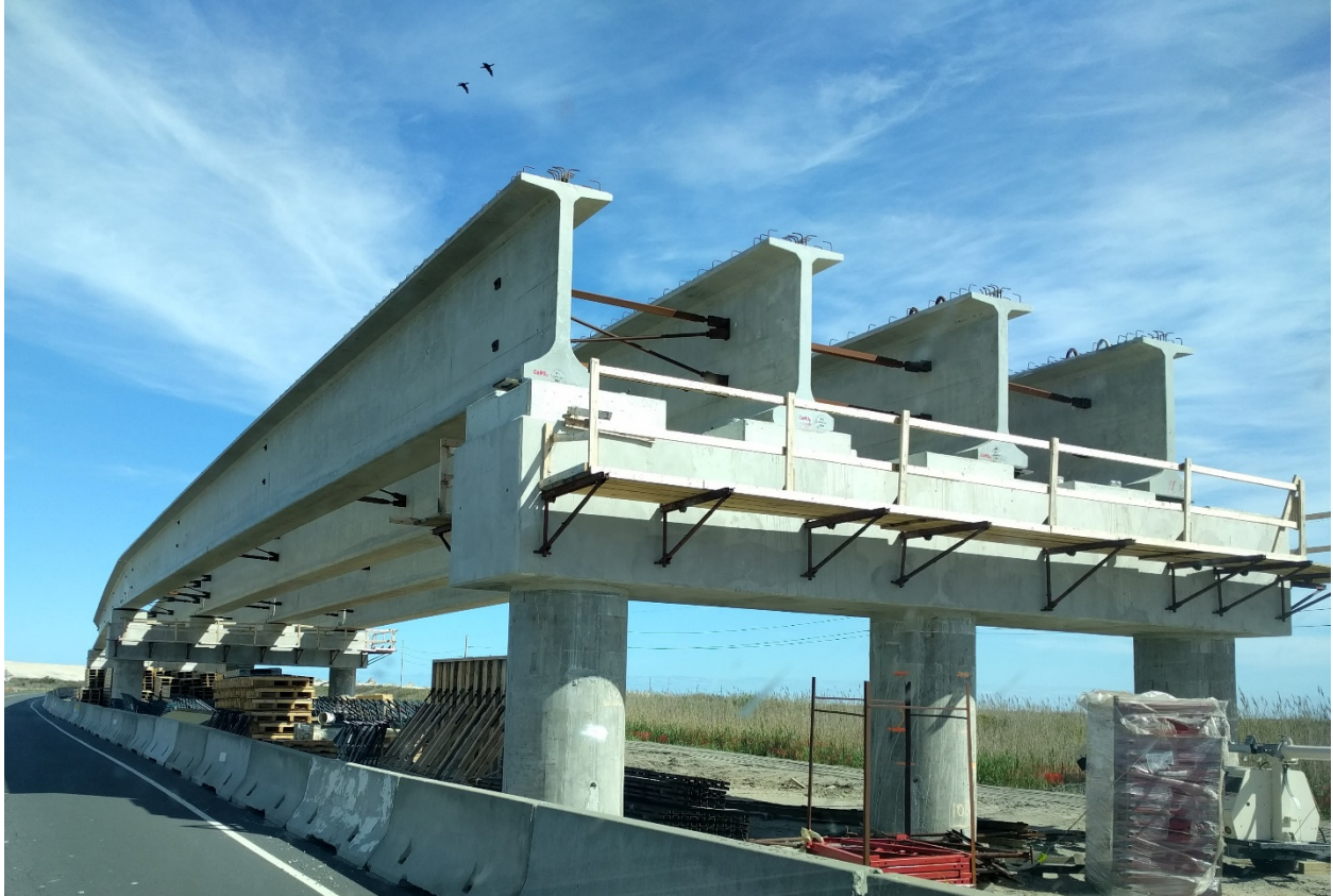
Fig. 7 South Approach Span construction, showing 96” deep precast concrete Florida I-Beam (FIB) girders supported by precast concrete bent caps and 54” diameter precast concrete cylinder piles.
