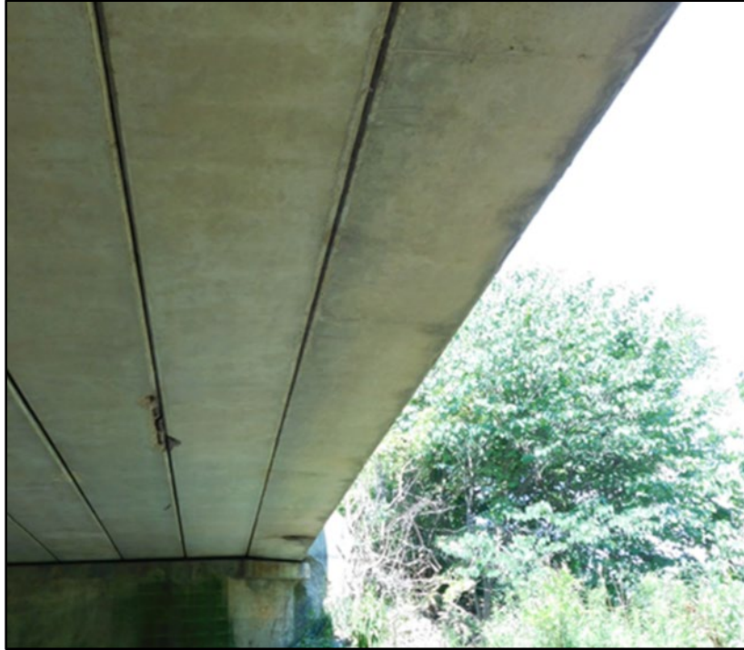
Fig. 13 Rotation of Exterior Beam (Clear Creek)
