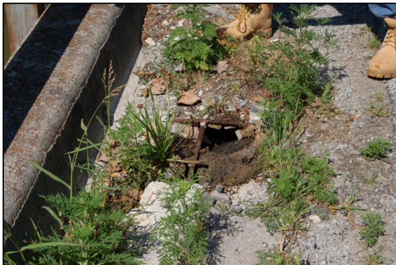
Fig. 14 Opening in Top Flange of Exterior Beam (Rock Creek)
