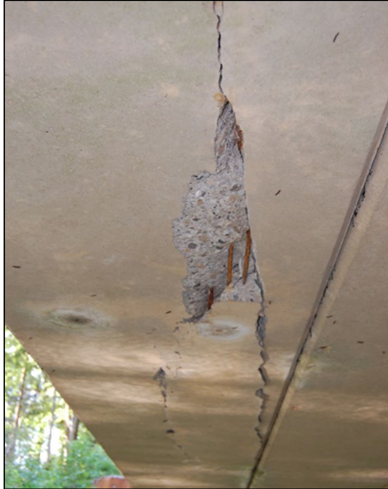
Fig. 10. Spalling and Exposed Strands (Yellow Creek)
