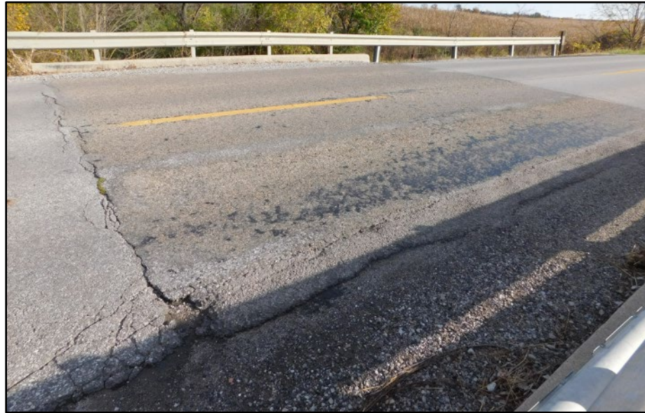
Fig. 15 Discontinuous Bituminous Wearing Surface and Reflective Longitudinal Cracking (Beal-Taylor Ditch)
