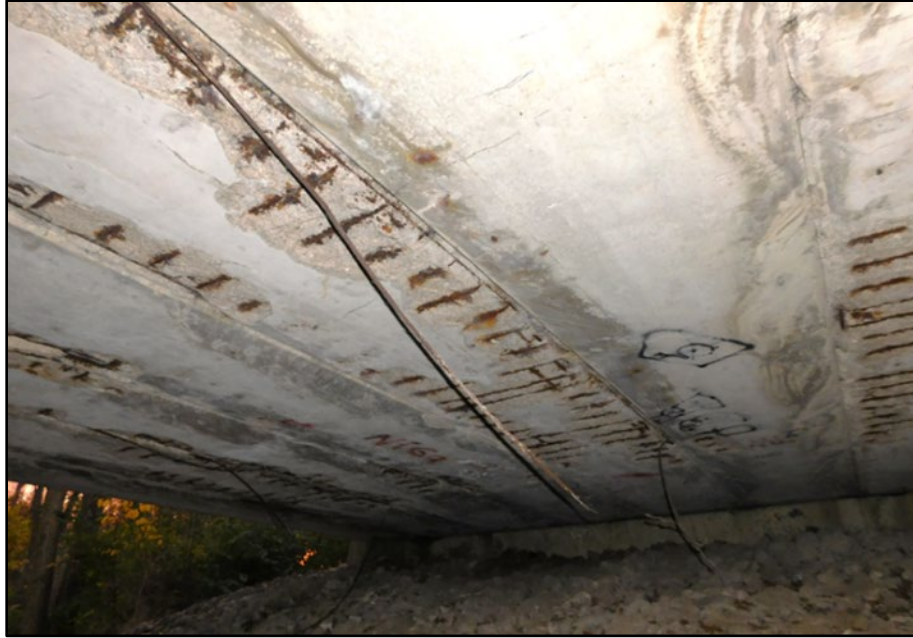
Fig. 11. Fractured Prestressing Strands and Corroding Shear Reinforcement (Main Street)
