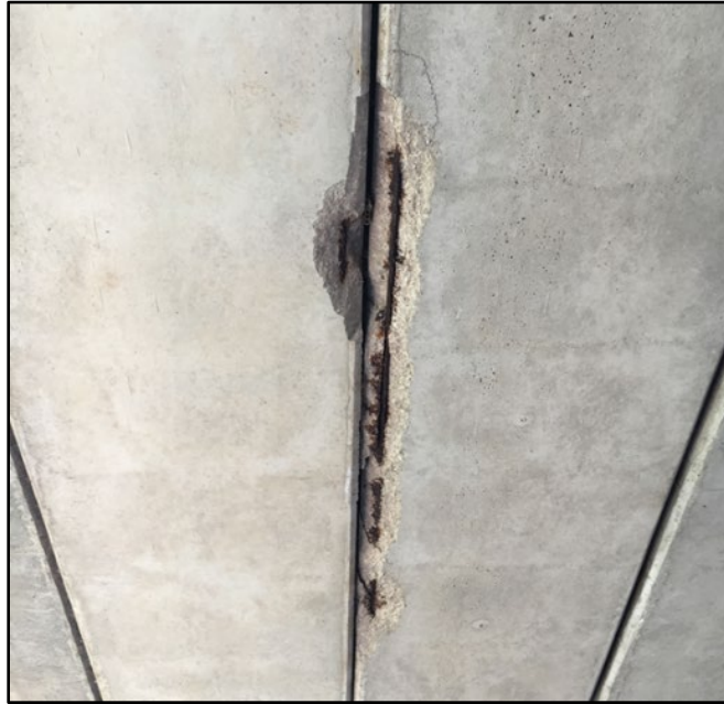
Fig. 9 Spalling Near Longitudinal Joint (Clear Creek)
