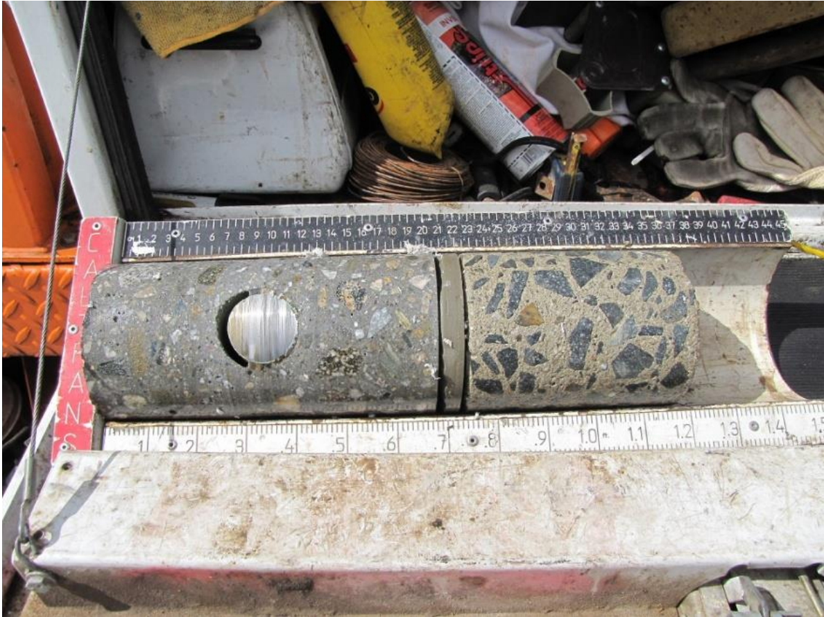
Fig. 8 Separation of Grout from Panel and Base
