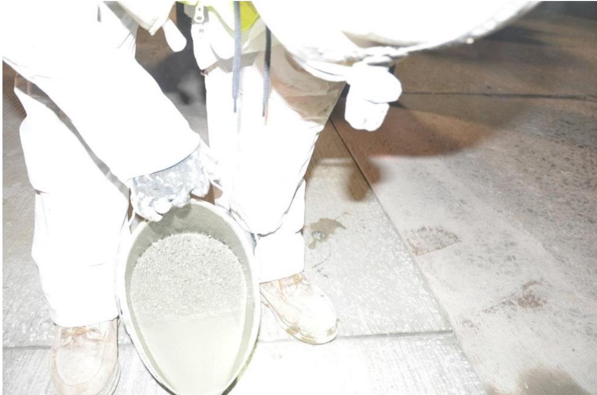
Fig. 9 Segregation of the Fill Material during Dowel Slot Backfill
