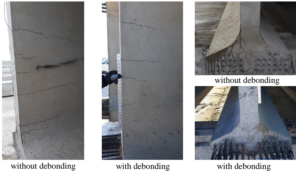
Fig. 11 Crack patterns of girders with and without debonding
