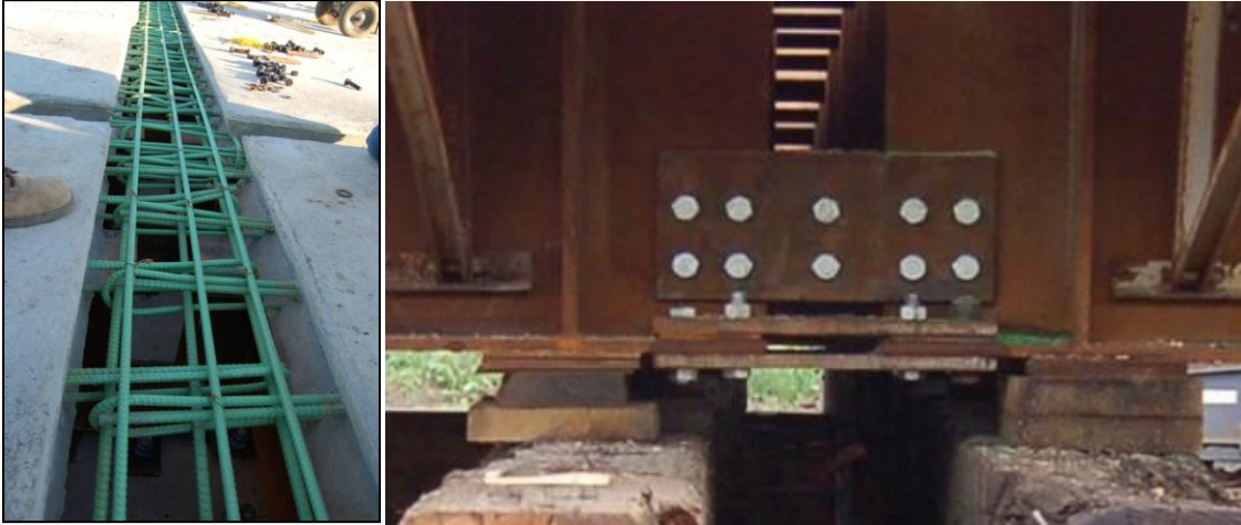
Figure 2 – Continuous Beam Modifications at Deck Top Reinforcement (Left) and Beam Bottom Flange (Right)
