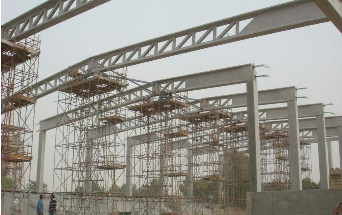
Fig. 4 Concrete trusses resting on the temporary supports before post-tensioning (Courtesy of e.Construct, USA, LLC)
