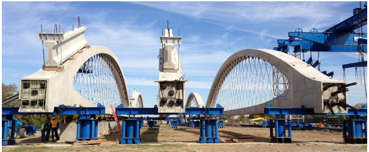
Fig. 8. Strongbacks Attached to Arch Ribs Prior to Stressing Hangers in Casting Yard
