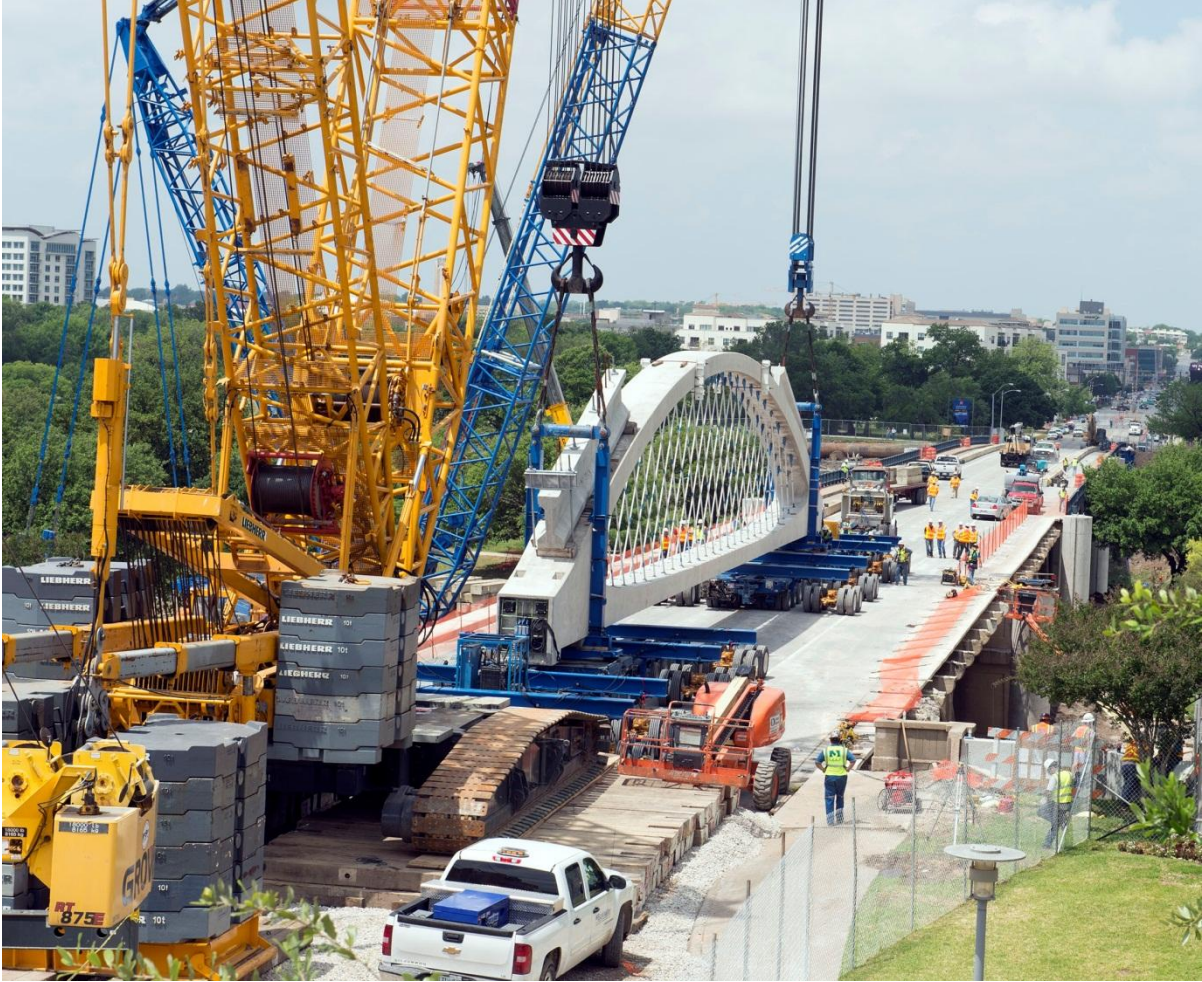
Fig. 13. View from Downtown of Two 600 Ton Cranes Lifting Arch from Existing Bridge
