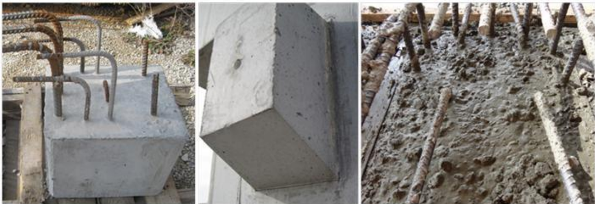
Fig. 1 Precast facility #1 corbel (left), corbel in place (center), precast facility #2 corbel (right).
