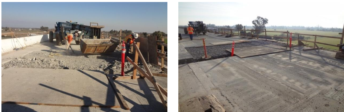
Fig. 2 Superstructure concrete grinding and demolishing at an in-span hinge (Bradley Overhead Replace)
