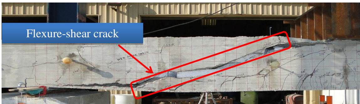
(b) Flexure-shear crack failure mode
