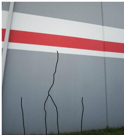
Figure 8 Vertical cracks in the wall panel (Cracks highlighted for clarity)
