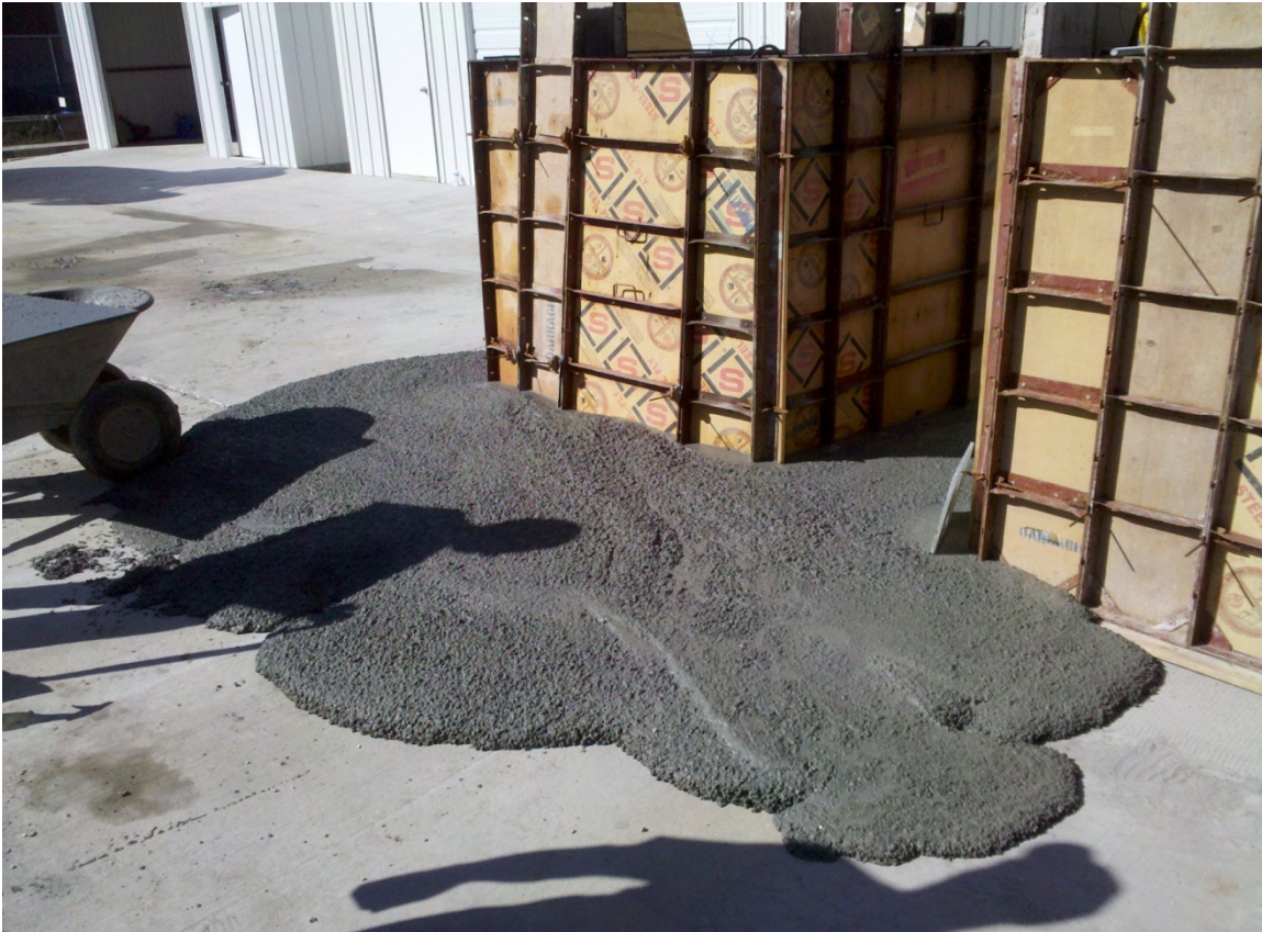
Fig. 5 Formwork Failure in Box Culvert # 1
