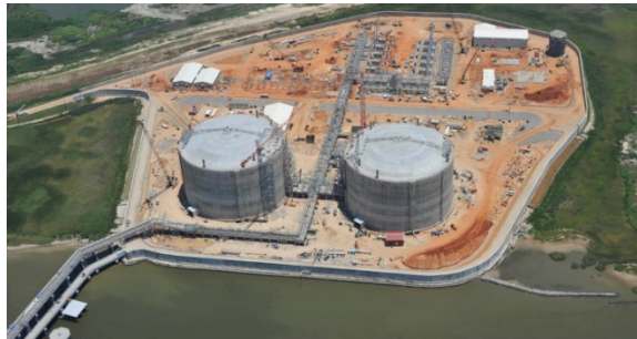
Fig. 1, A typical LNG receiving terminal showing both the marine berths for the LNG carriers and the LNG storage tanks and associated regasification equipment under construction. Photo courtesy of Baker Concrete.
