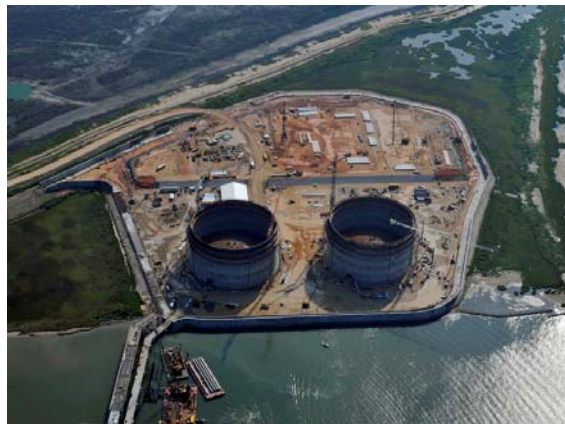
Figure 3. Conventional LNG storage tank under construction. The secondary containment roof has not yet been constructed in this photo. Photo courtesy of Baker Concrete.
