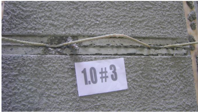
Figure 14: Pull-out of the tie from the concrete
