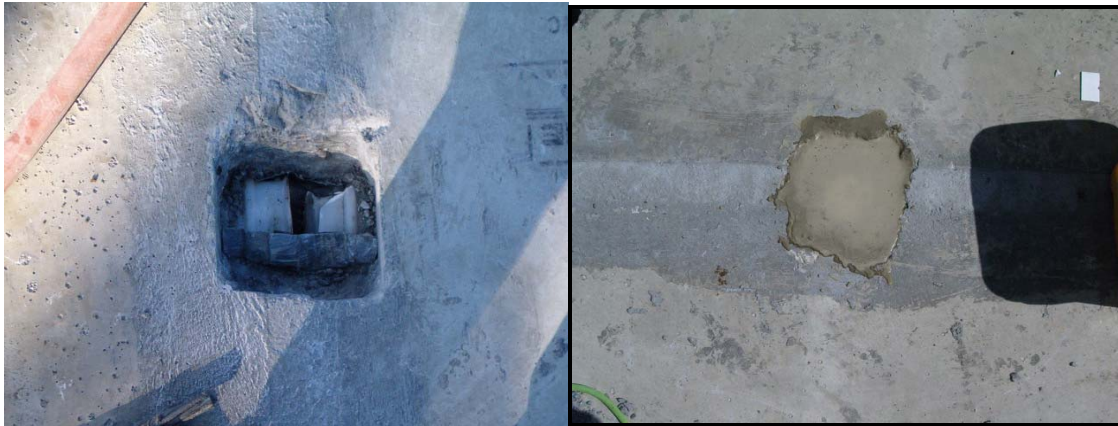
Fig. 11 - Misaligned Ducts in Handhole
