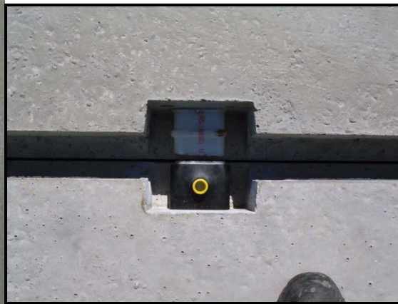
Fig. 10 - Aligned Ducts in Handhole
