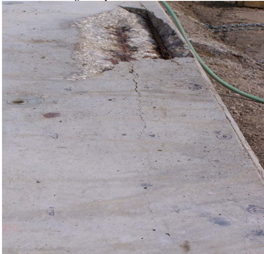
Fig. 7: Exposed Strands of Beam 4
