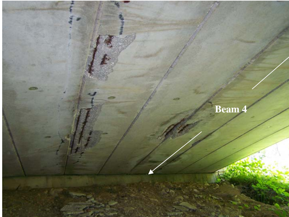
Fig. 6: Exposed Strands of Beam 4
