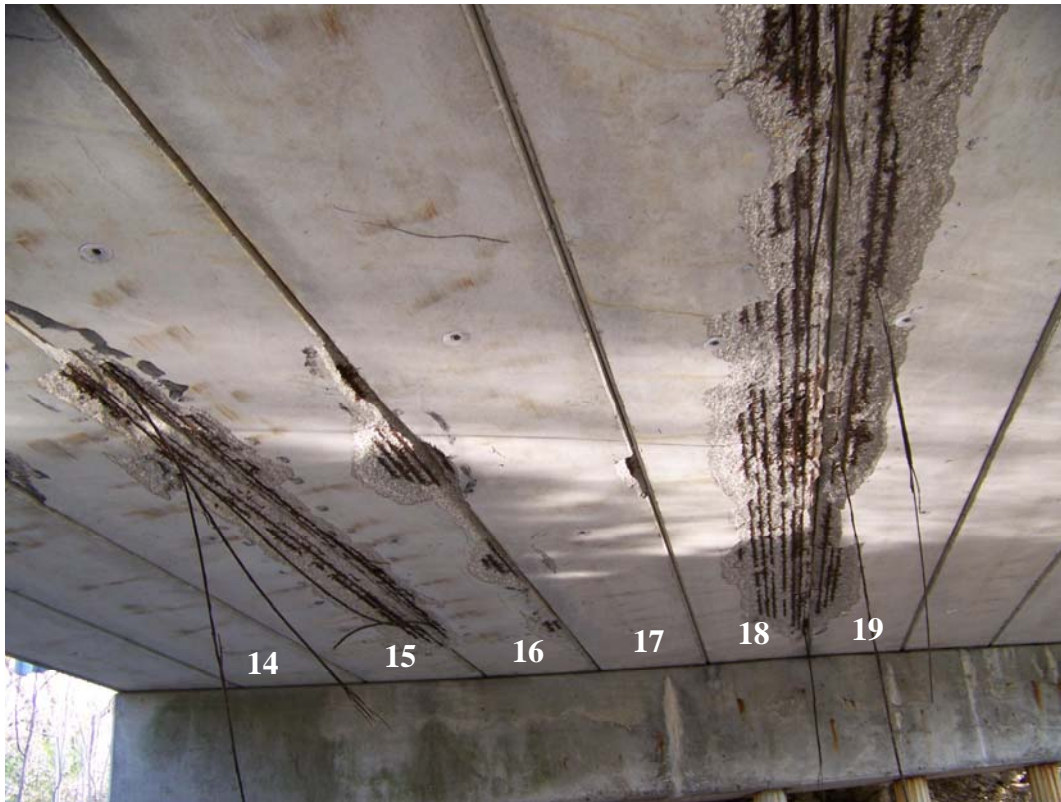
Fig. 8: Exposed Strands of Beams 15 and 18
