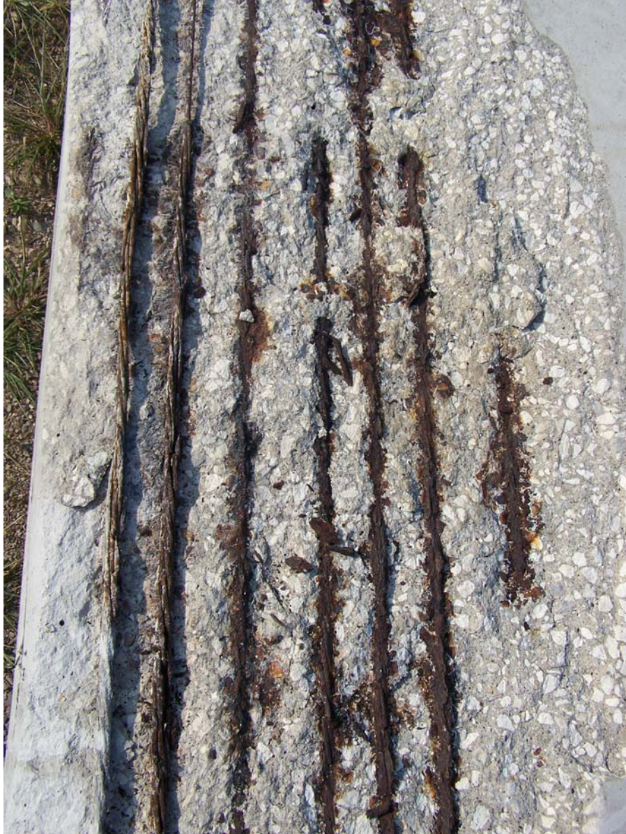
Fig. 9: Exposed Strands of Beam 18
