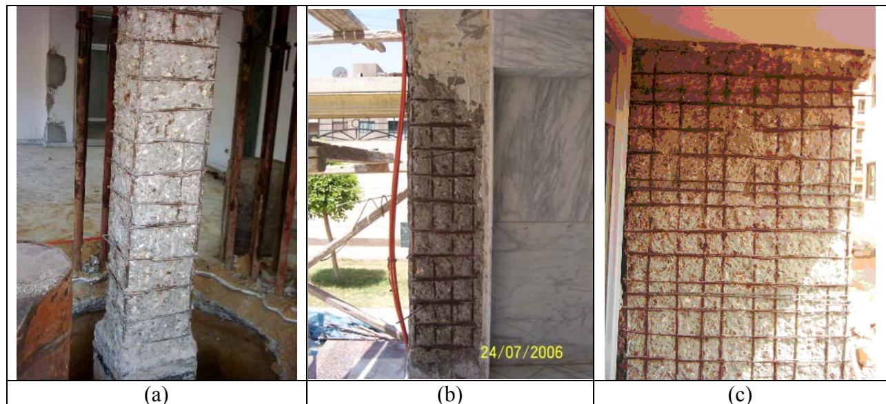
Fig. 1 Corroded Steel reinforcement (a) interior column, (b) exterior column, and (c) exterior column
