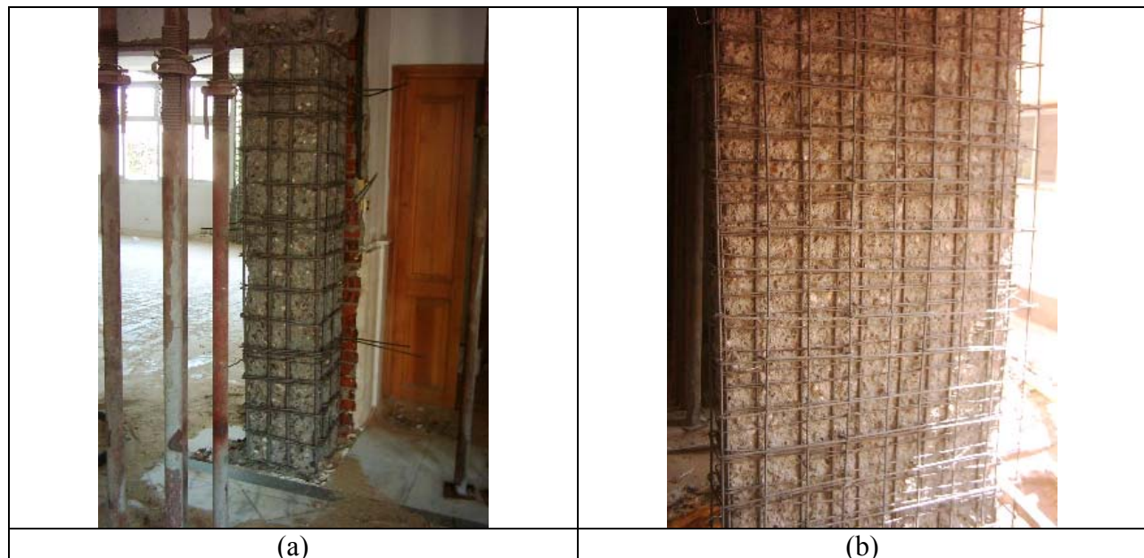
Fig. 2 Sand blasted steel and new steel (a) interior column, (b) exterior column
