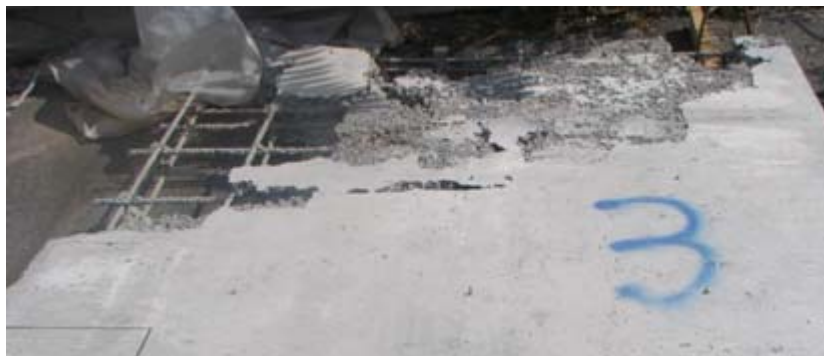
Figure 4. Poor filling and flow of Mix W-3 in wall panel
