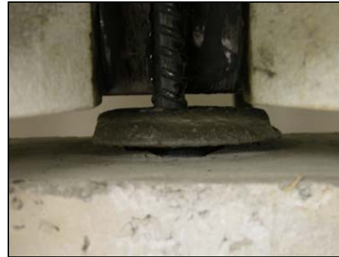
(e) Slippage Failure
