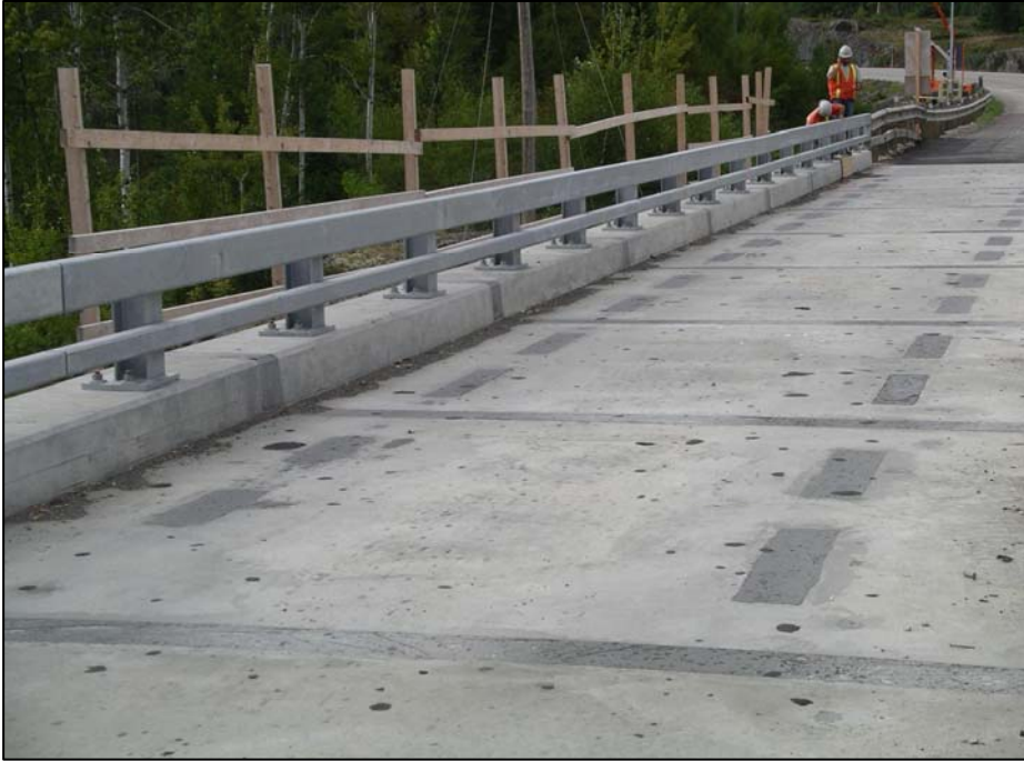
Fig. 10 CN Overhead at Rainy Lake Bridge with precast deck panels and UHPC joint fill
