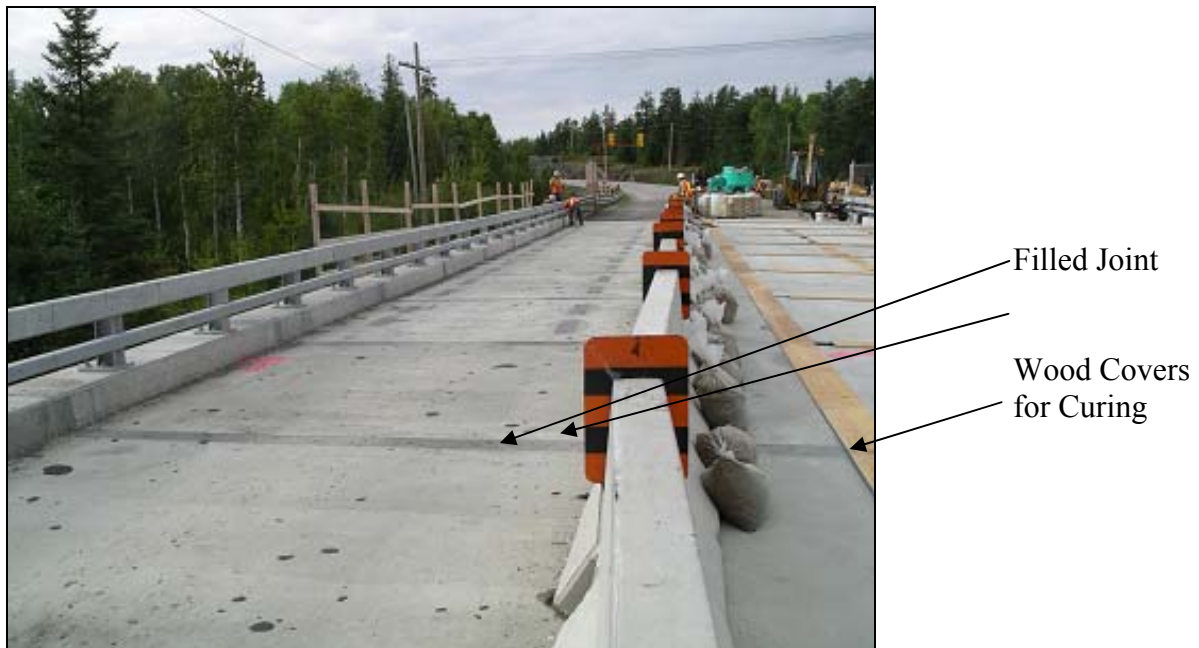
Fig. 7 Maintaining one lane open to traffic at all times during the deck reconstruction
