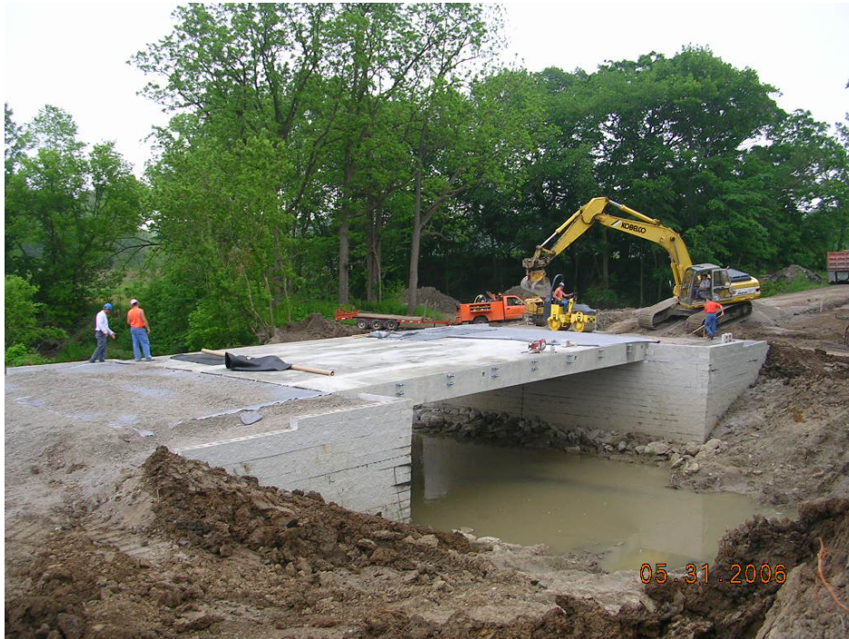
Figure 11. Integration of Approach Way for the Glenberg Bridge – Next Day After Beam Placement
