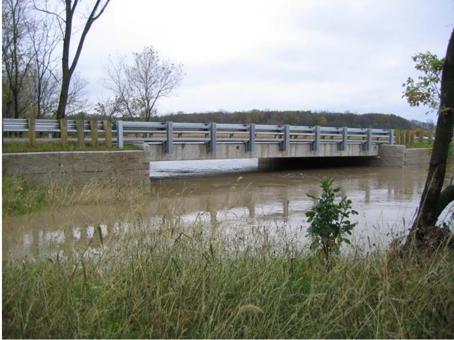
Figure 12. Completed Glenberg Bridge Above Flood Waters. (note: wood guard rail posts should never be used in GRS applications)
