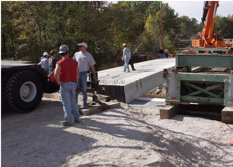
Figure 9. Placement of Concrete Box Beams Directly on the GRS Abutment (note absence of concrete footing)
