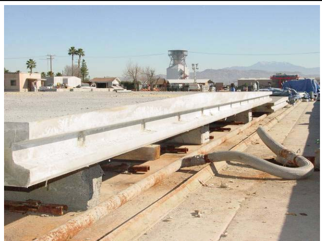
Fabrication of panels for the California demonstration project showing the unique cross-section required to achieve the change in cross-slope in the finished surface.
