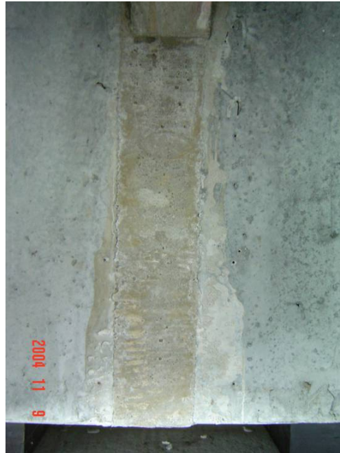
Figure 15 Low Side, Little to No Cracking
