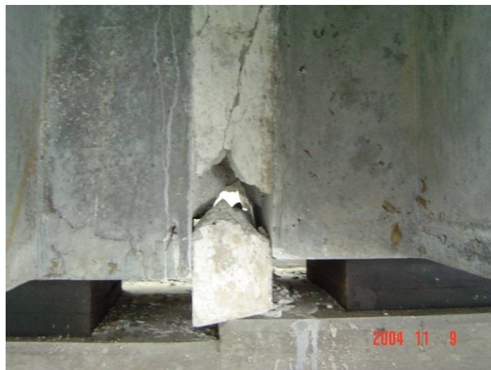
Figure 14 High Side Cracking
