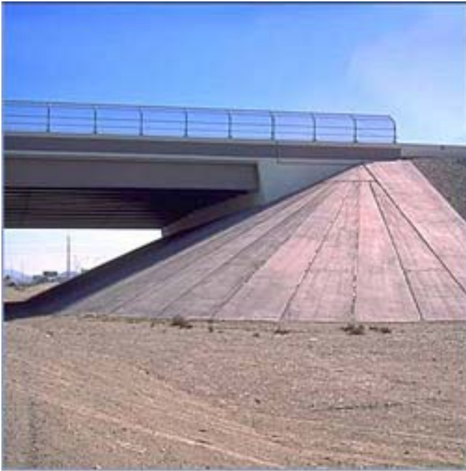
Color can add a finishing touch to bridge abutments and related structures.
