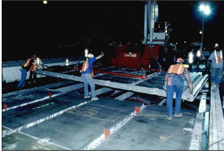
Fig. 2 Full-depth deck panels on Tappan Zee Bridge over Hudson River in New York
