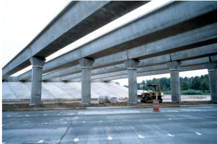
Fig. 5 Precast piers at Louetta Road Overpass on State Highway 249 near Houston, Texas
