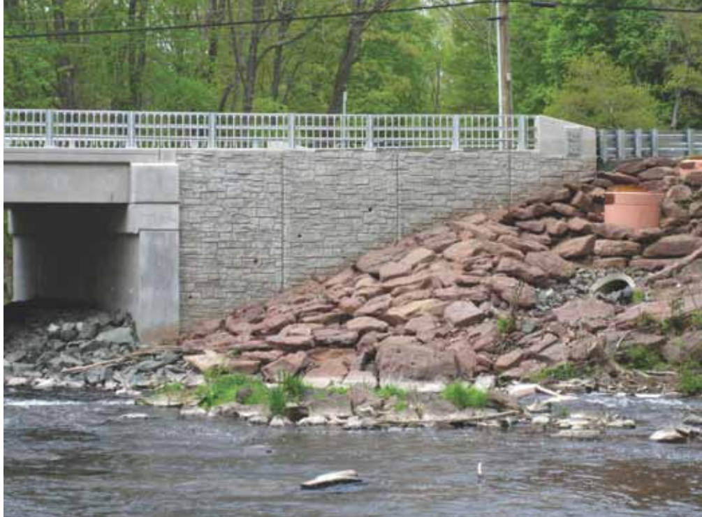
Most of the components of the bridge are shown: box beams, abutment and wingwall panels, cheek walls, and the bridge seat beam with its extended lip covering the horizontal joint with the abutment panels. Photo: Hoyle, Tanner & Associates Inc.
