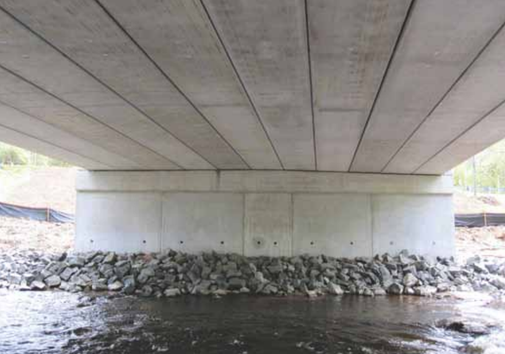
The underside of the South Maple Street Bridge. Photo: Hoyle, Tanner & Associates Inc.
