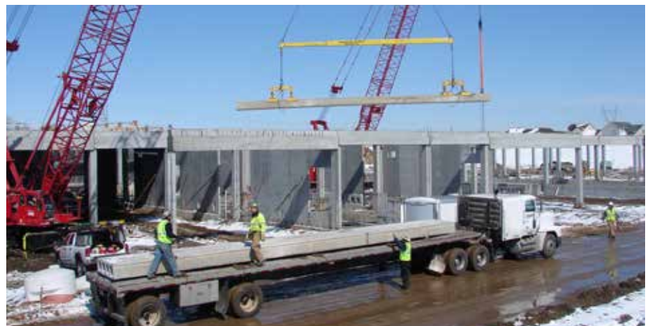
Owner: Next Tech • Architect: Corgan Associates • Engineer: L.A. Fuess Partners, Inc. • General Contractor: M.A. Mortenson Construction • Photo Credit: Jason Becker, Molin Concrete Products • Location: Chaska, MN
