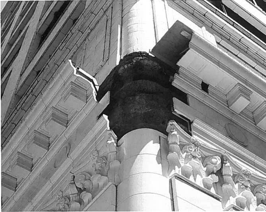
During restoration of One North State Street in Chicago, rubber molds were used to replicate existing elements and duplicate the terracotta coloring and texture.
