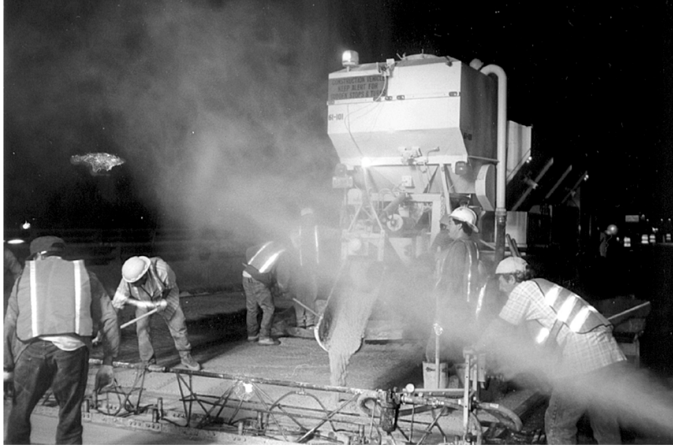
FIGURE 1. LMC-VE overlay is placed and consolidated on middle lane of bridge on Rte. 620. A fog spray humidifies the air behind the screed to prevent plastic shrinkage cracking.
