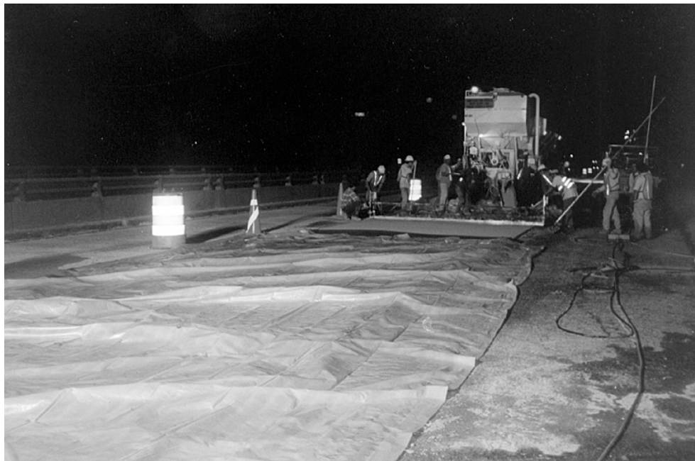
FIGURE 2. LMC-VE overlay is quickly covered with wet burlap and polyethylene to provide a moist cure. The overlay can receive traffic in as little as 3 hours.
