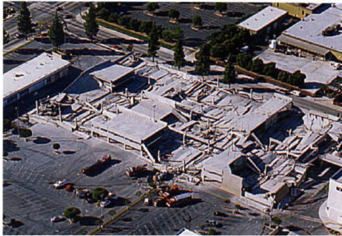
Fig. C-2: Precast parking structure collapse, 1994 Northridge Earthquake (Courtesy: Los Angeles Times ).
