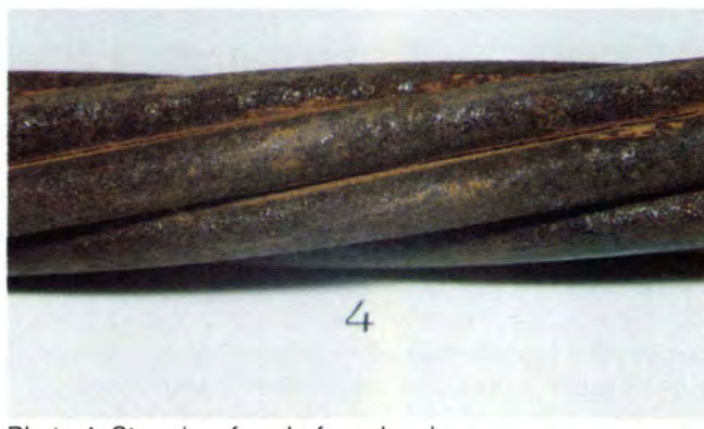
Photo 4. Strand surface before cleaning.
