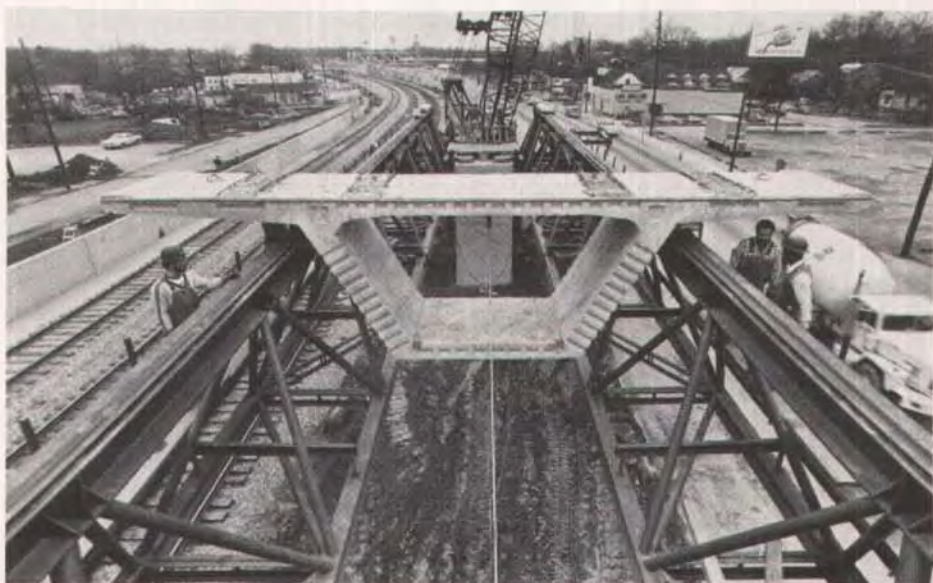
The wings of the segment rest on movable supports that are on the top flange of the trusses. Segments were winched into place in the span.
