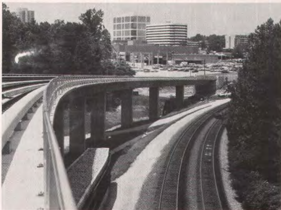
Approximately 370 ft (113 m) of the second elevated structure had to be built over an operational railway line.
