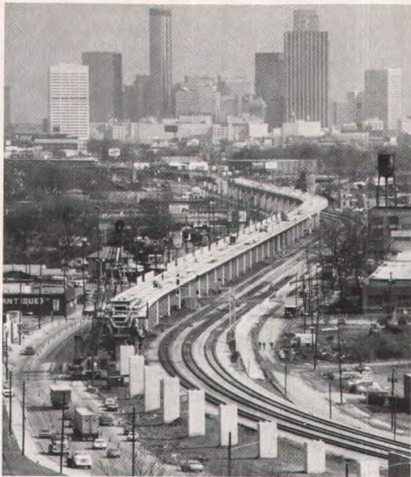
Panoramic view of Atlanta's MARTA 360 rapid transit project. Precast prestressed segmental construction (span-by-span method) enabled the contractor to place four spans of up to 100 ft (30.5 m) in length per week.
