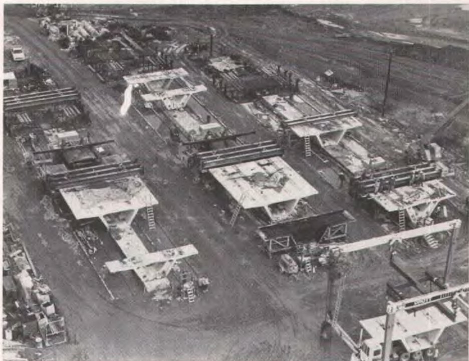
Precast yard for the box girder segments was located two blocks from the first elevated structure. Long-line casting beds are first in the United States for full span.
