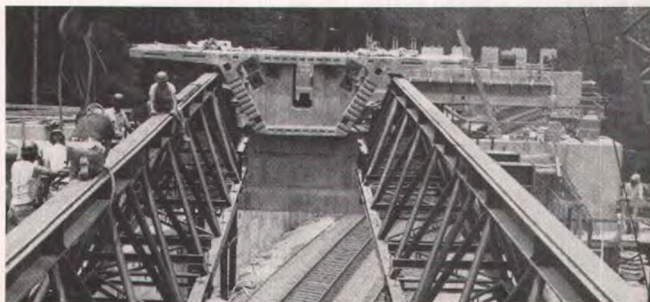
One of the twin triangular trusses being moved. Spans are 70 to 100 ft (21 to 30 m) at this particular place in construction.
