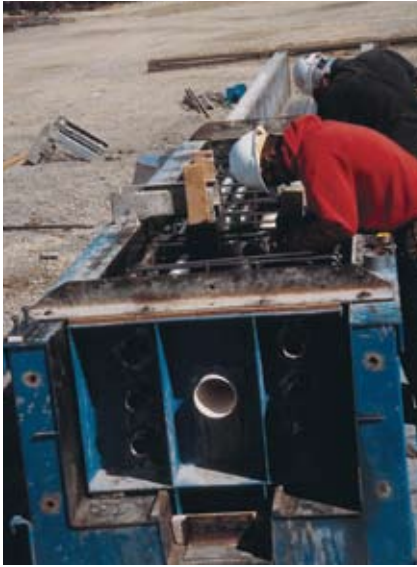
A moment-frame beam form illustrates the center PVC duct that holds the prestressing tendons and the six corrugated tubes for the mild steel bars used in the hybrid system.
