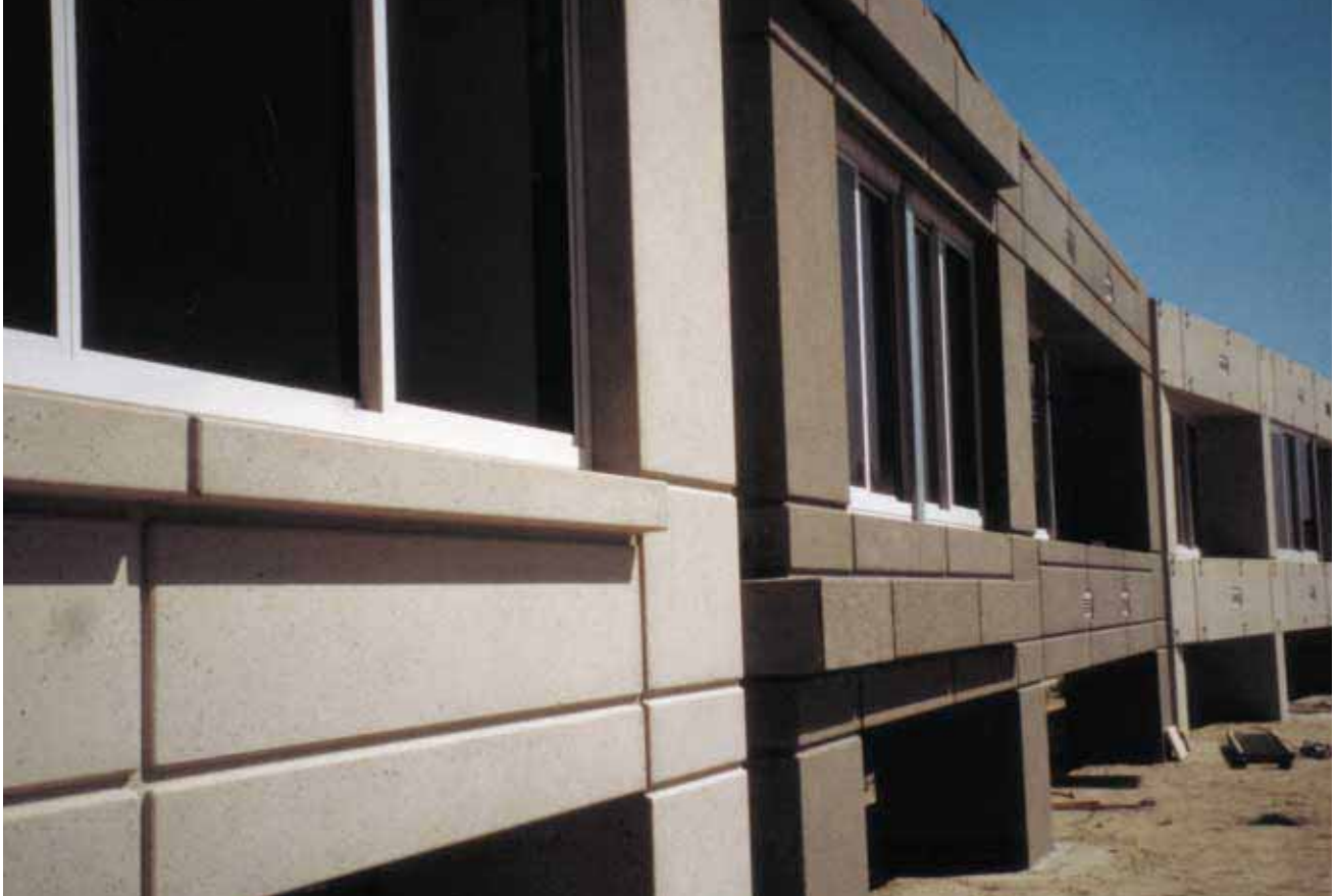
Three full-size mock-up panels were produced for the Mission Apartments project to replicate the different finishes and textures to be incorporated.
