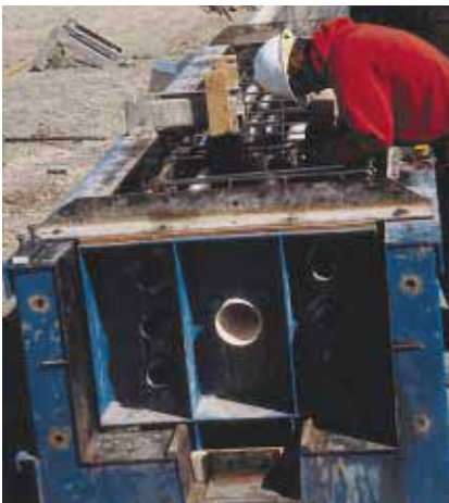
This moment-frame beam form shows the center PVC duct that holds the prestressing tendons and the six corrugated tubes for the mild steel bars used in the hybrid system.
