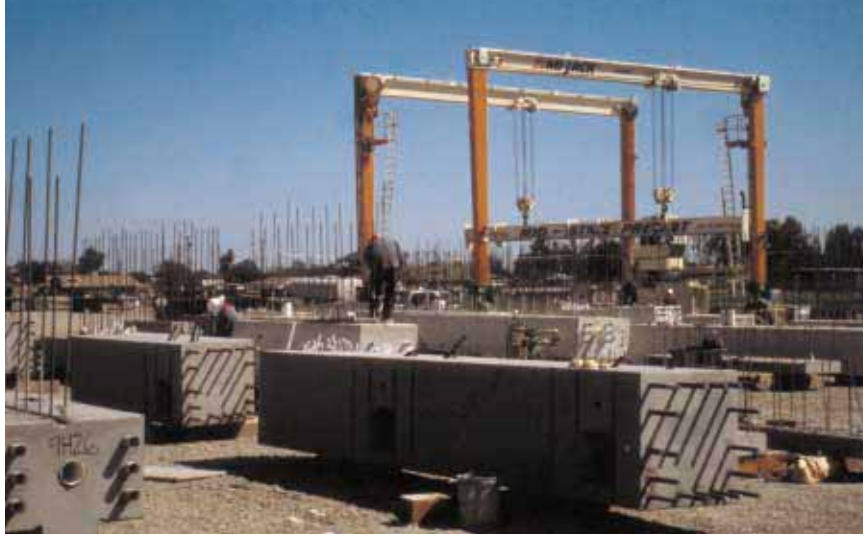
Beams cast for the project are being stored in the precaster's yard in Corcoran, Calif., until needed to ensure erection moves smoothly and rapidly once the site is ready.
