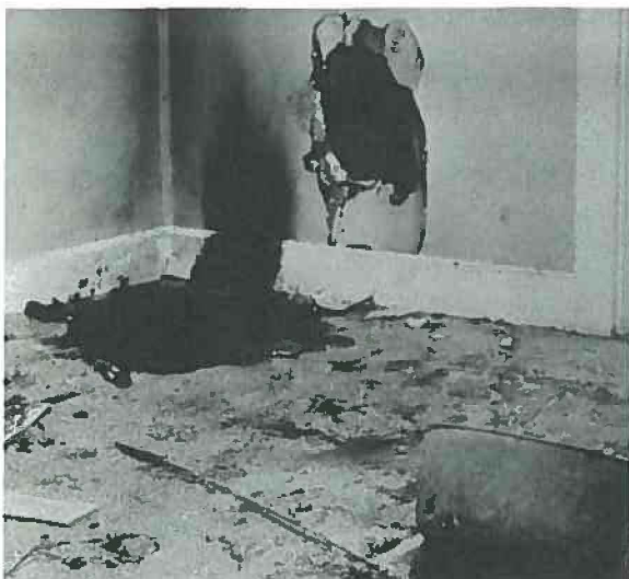
An unsuccessful arson attempt. The gasoline can and shredded papers are good indicators of arson. The hole was punched into the wood-frame wall to facilitate fire spread. (Photograph from Arson: Origin and Cause Determination, Part A . Copyright © 1979 National Fire Protection Association, Quincy, Massachusetts. All Rights Reserved.)
