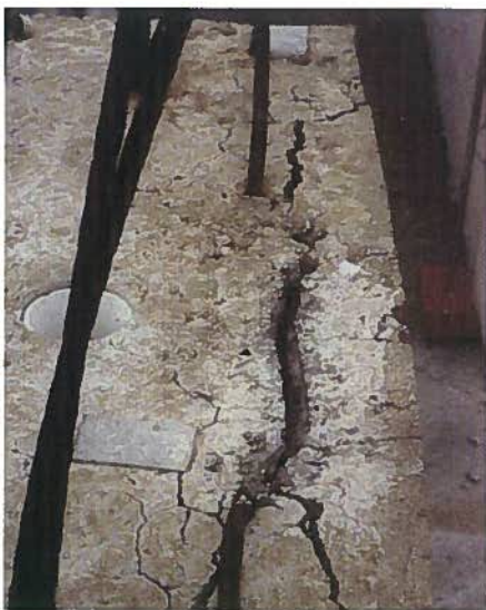
Fig. H. Opening of the shrinkage crack. Courtesy of Kevin Pruski, Texas DOT.
