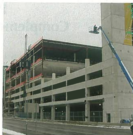
A two-hour fire rating was achieved between the parking and retail levels by using double tees.
