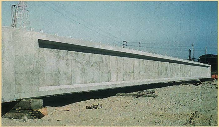
Fig. 6. A 105 ft (32 m) roof girder for Woodrow Wilson High School in Tacoma, circa 1956.
