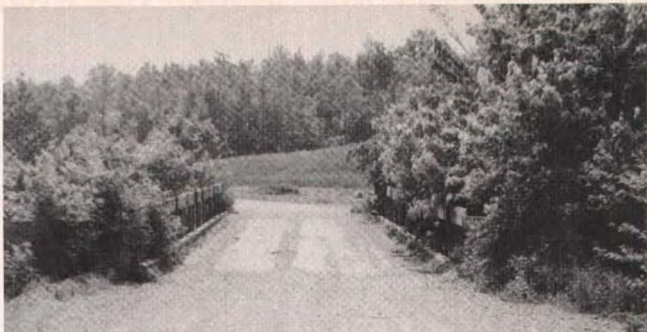
Old, narrow, single lane structure.
