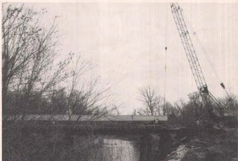
The old structure, with the assistance of a crane, permitted new beams to be stacked adjacent to the old structure.
