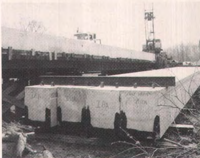
The new beams were stacked adjacent to the old structure because two cranes were required for final beam placement.
