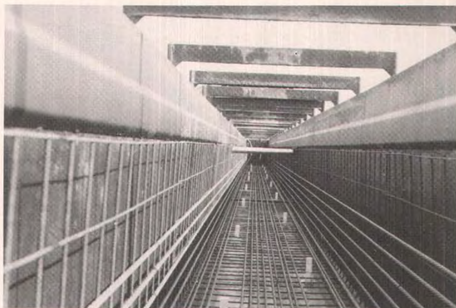
Interior of forms showing placement of strands and reinforcing steel for bottom and sides.
