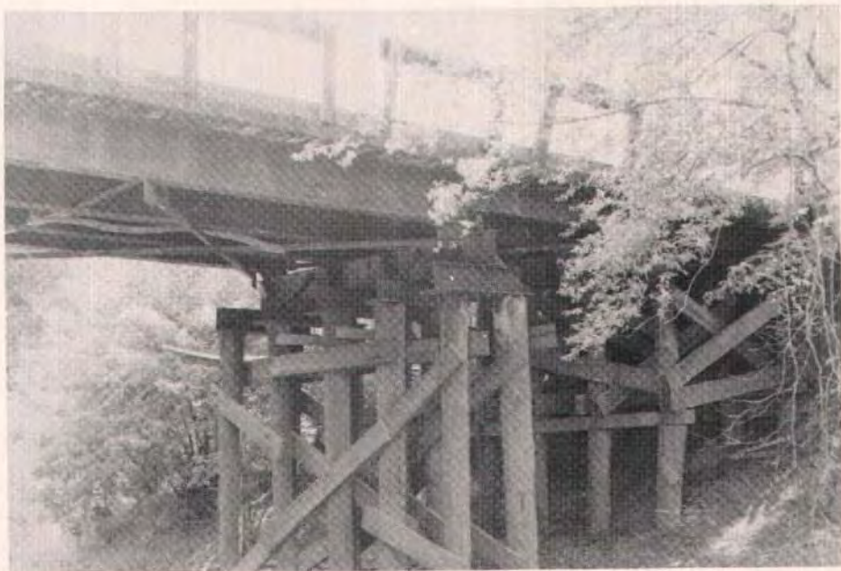
Deteriorated east abutment/pier complex of old bridge.
