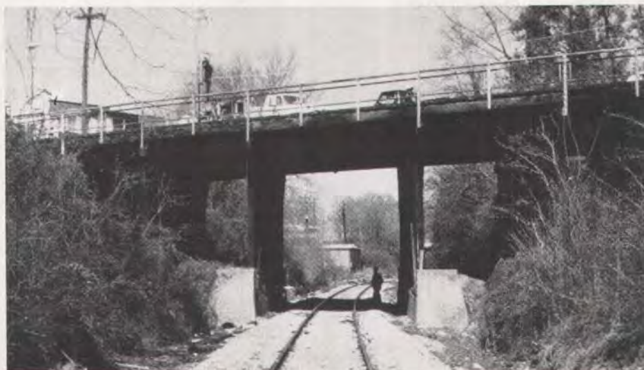
Fig. 1. Old deteriorated highway bridge.
