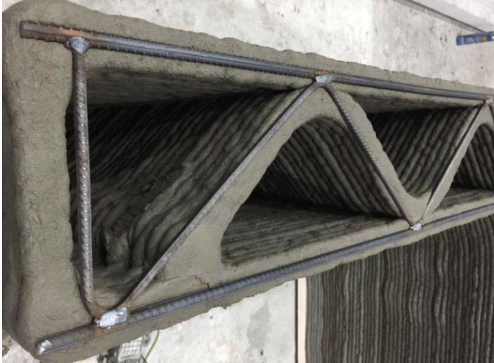
Fig. 7: 3D printed cassette during fabrication. Steel rebar truss was placed manually between the 3D printed concrete layers
