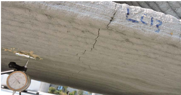
Fig. 10: cracking pattern at the mid span during testing.
