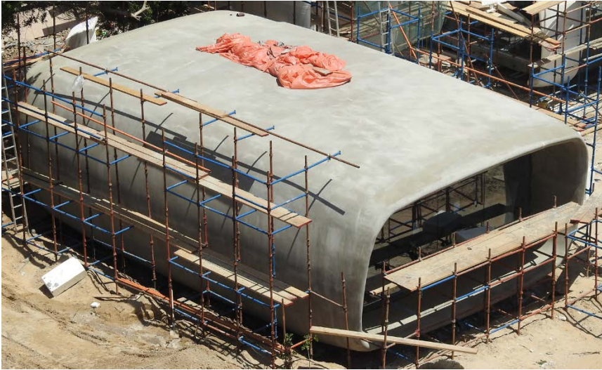
Fig. 21: 3D printed office during applying the external finishing. Insulation was attached from outside and external finishing was applied.
