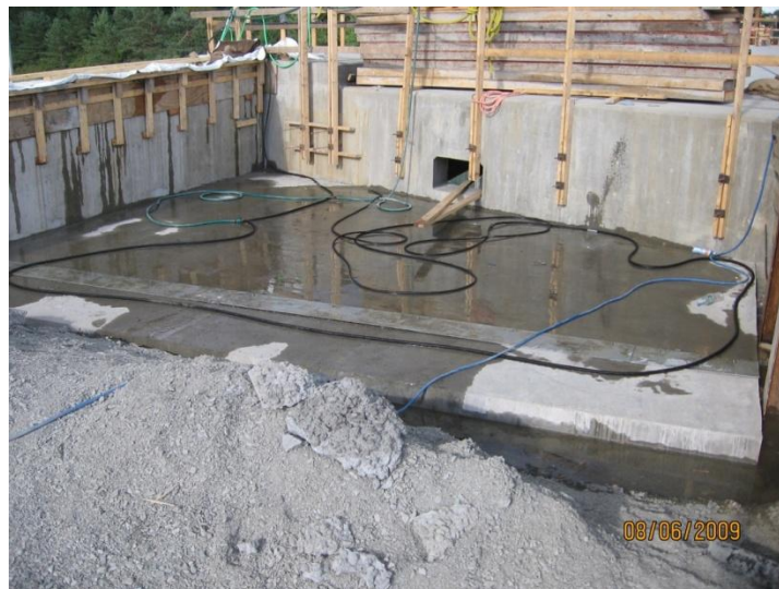
Approach Slabs: No Bond to Wingwall at the Slab Level
