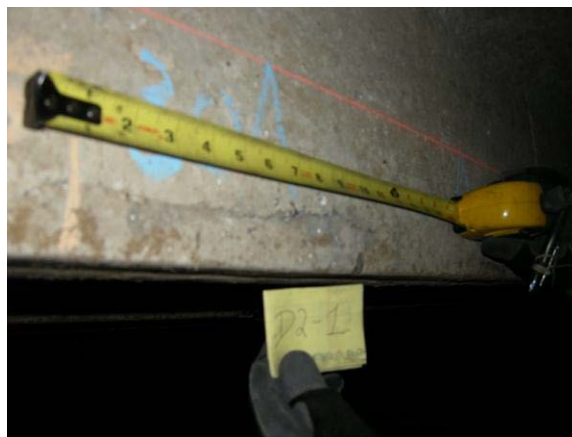
Figure 4 Cracking near location of prestressing strand
