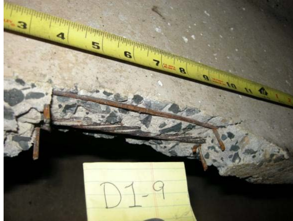
Figure 3 Spall and exposed prestressing strand
